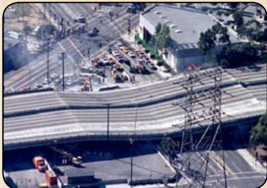
Part of Interstate 10 west of downtown Los Angeles collapsed in the shaking of the 1994 Northridge earthquake.
